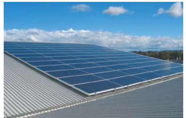
Medium-sized system using multiple inverters.
