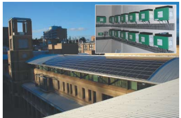
A medium-sized system using multiple inverters. (7)
